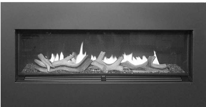
Figure 46 - Burner Flame Appearance
