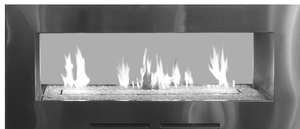
Figure 9 - Incorrect Burner Flame Pattern caused by port blockage
