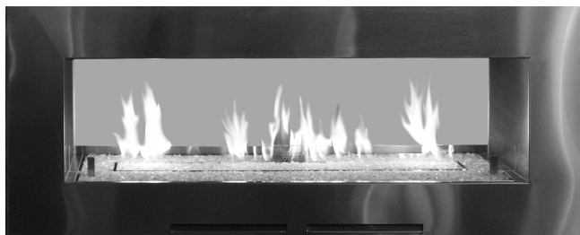
Figure 9 - Incorrect Burner Flame Pattern caused by port blockage
